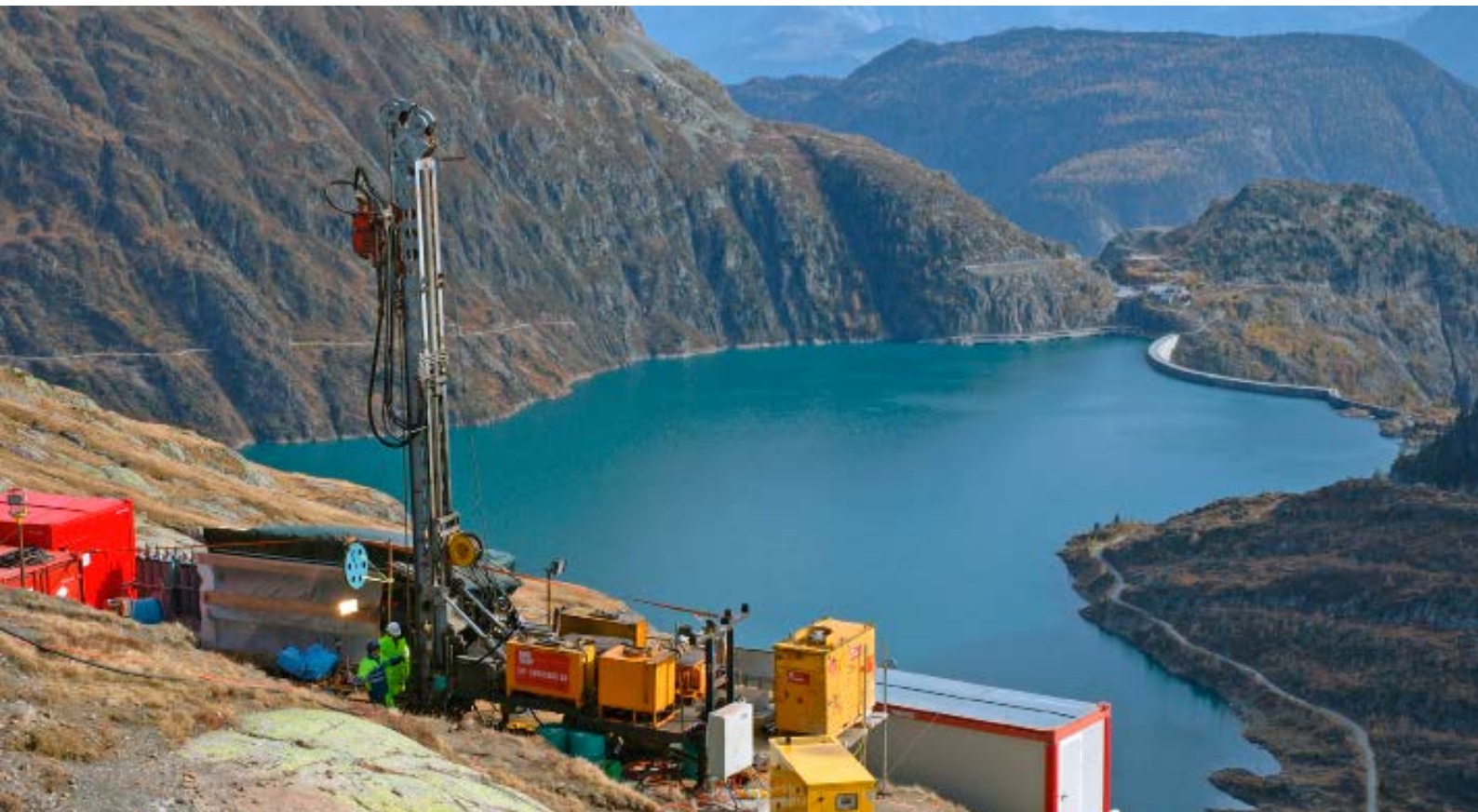
Planned pump-storage scheme Nant de Drance, Emosson, Canton Valais: hydraulic and rock mechanics borehole tests
