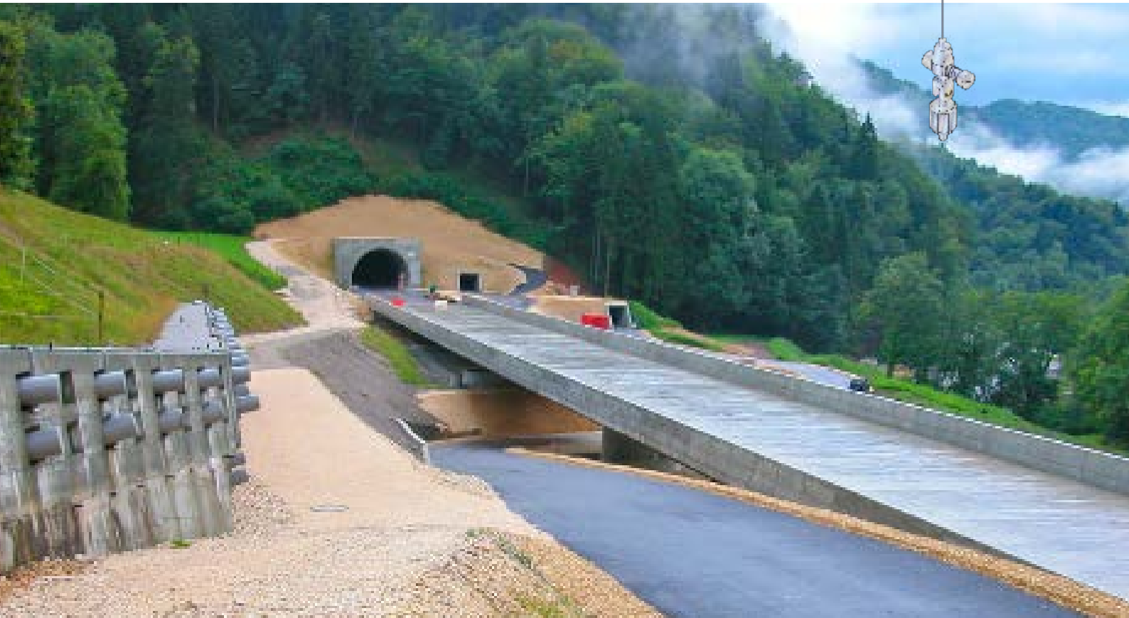
Highway A16 Transjurane, New development, Section Roches-Moutier, Canton Berne: Trivec measurements in a pile wall
